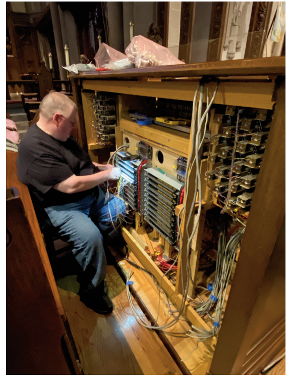
Ed Helgerman installs the console input boards and prepares over 800 wires to be individually attached to quick connectors that will allow for ease of access for future service work.
